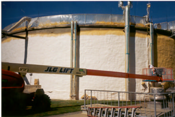
2" OF 3# SPRAY POLYURETHANE FOAM PROTECTED WITH 50 MILS POLYSHIELD SS-100™ ON SEWAGE DIGESTER TANK, SIDEWALLS AND ROOF
